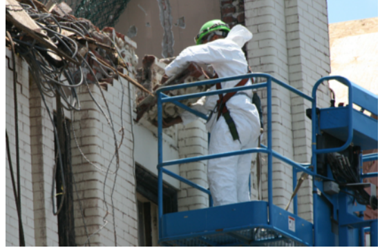
Salvage of the 1898 terra-cotta Green Man during demolition of the Ross Building, June 2008.
